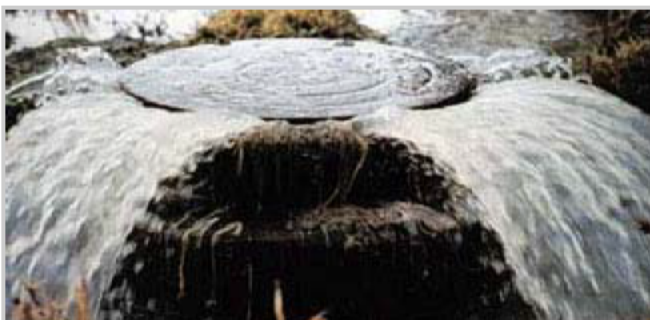
Photo of a sewer overflow
