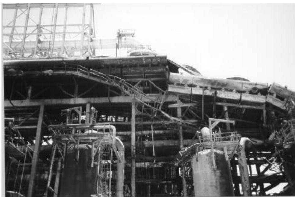
Figure E-4: Photograph of explosion and fire damage at OP-III as seen from north side of pipe rack, looking upward.
