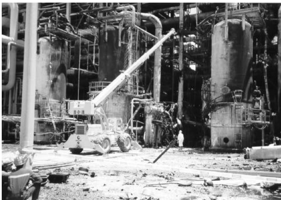
Figure E-6: Photograph of explosion and fire damage in the area of the PGC fifth stage suction and discharge drums (viewed from the north). The man in the lower center provides a reference to the scale of the surrounding structures. The failed check valve was located behind the drum to the man's right.
