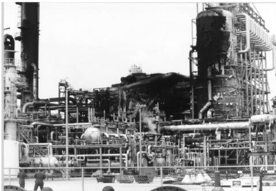
Figure E-1: Photograph of the damage resulting from the explosion and fire at Shell Olefins Plant Number 3 (view from west of blast area). Note the heavy structural damage in the rear center of the photograph.
