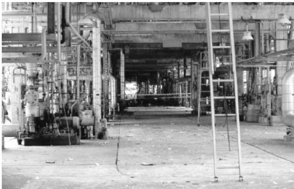
Figure E-5: Photograph looking down pipe alley (passable area underneath pipe rack) where explosion occurred.
