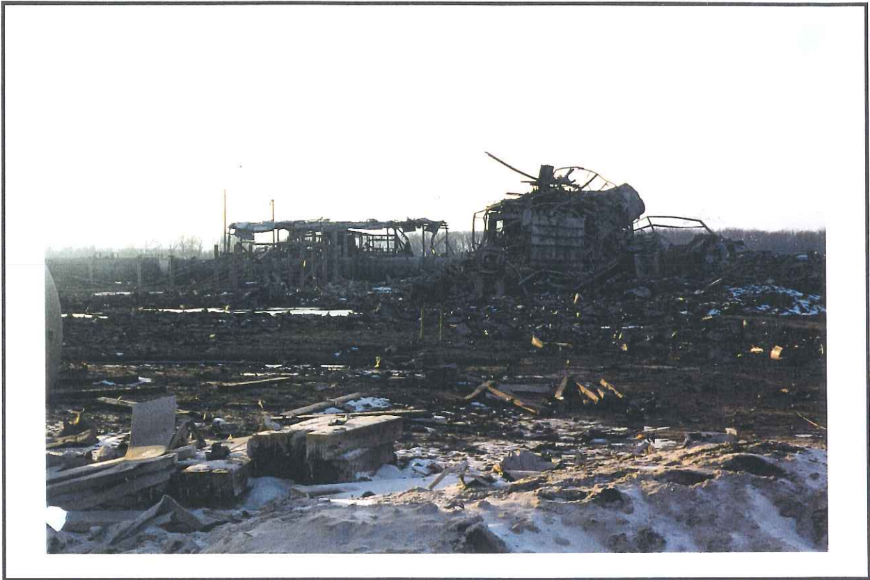
Photo 3 - 1 AN Plant Area After Explosion
