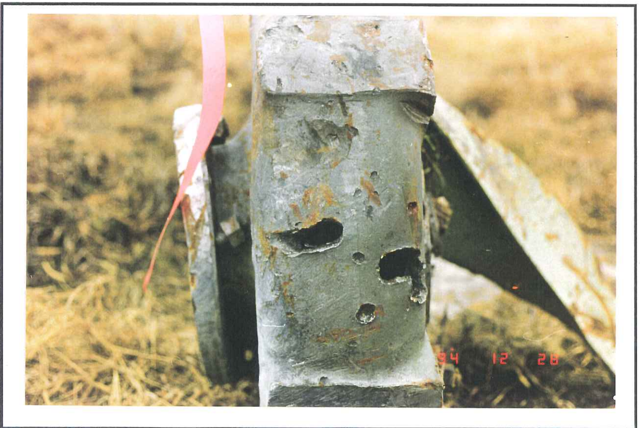
Photo 8 - 6 416J External Damage
