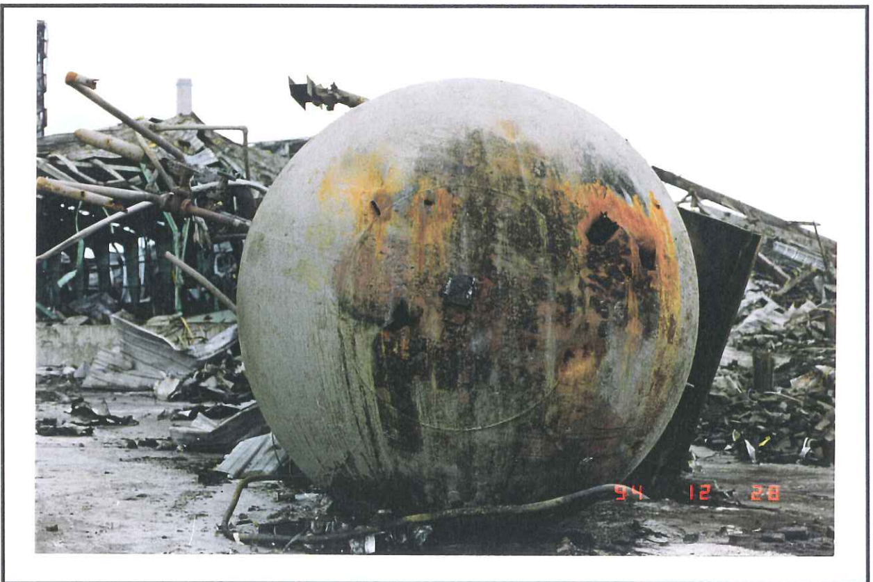
Photo 8 - 13 Ammonia Bullet Tank Damage
