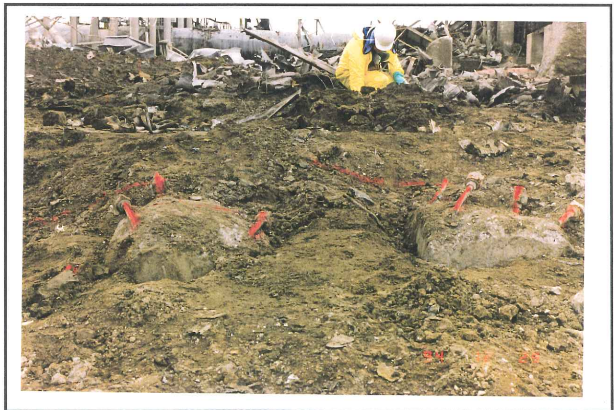
Photo 8 - 2 83% Product Pump Pads
