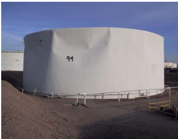
Tank Damaged by Negative Internal Pressure (Vacuum)
