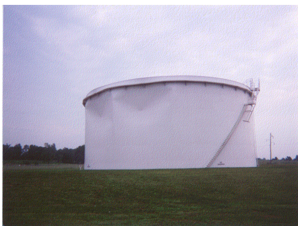
Tank Damaged by Tornado Winds
