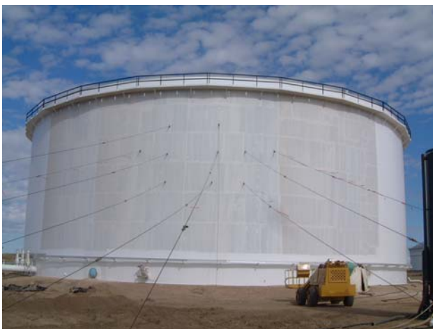
Tank Damaged by Wind (After Pulling Out Dents)
