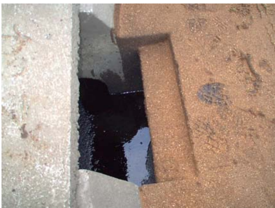
Fig. 7 – Rainwater sewer inlet.
