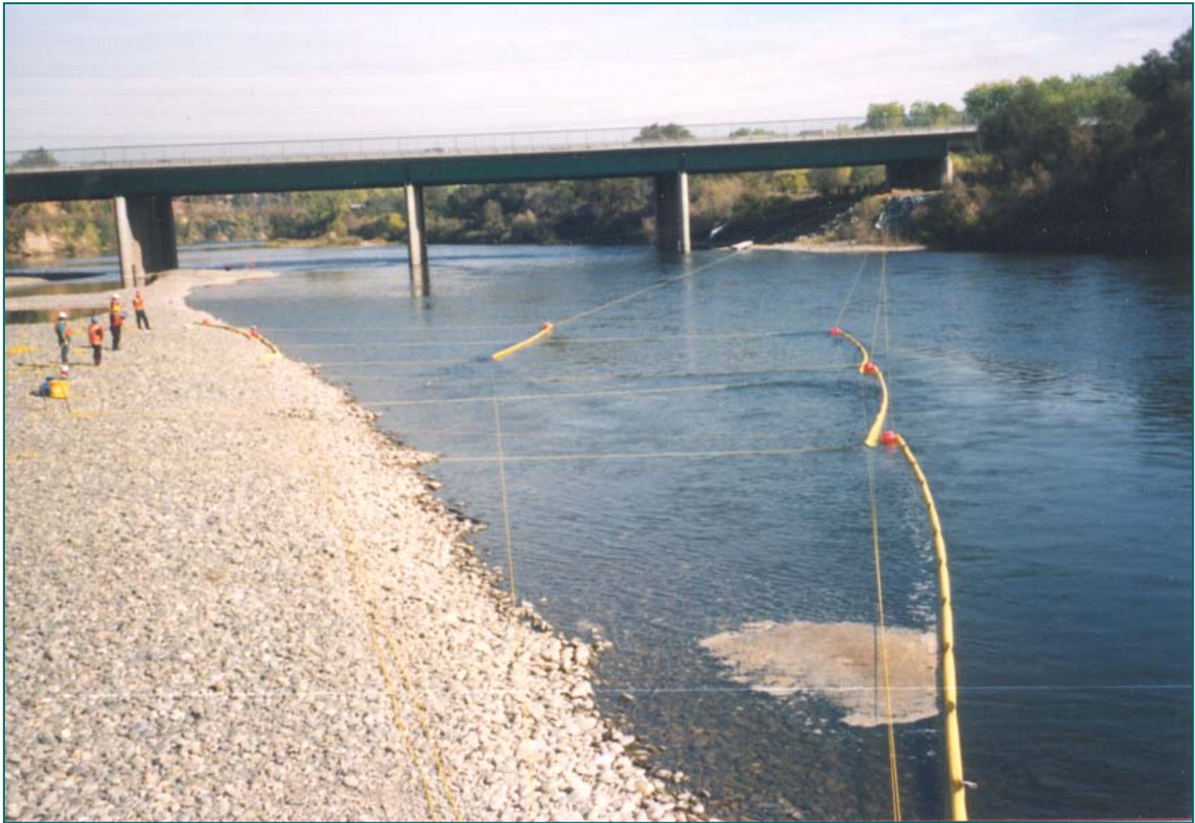
No. 4 - Boom Being Deployed - Bank to Bank Rope Anchor System American River - California
