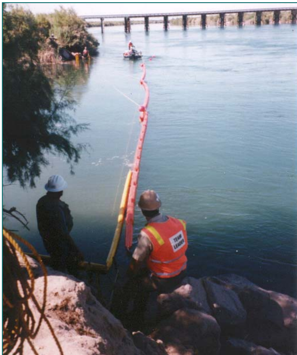
Bridge to Bank Rope Anchor System Boat deploying Rope Lead to Column "D" Ring & Shore Colorado River - California
