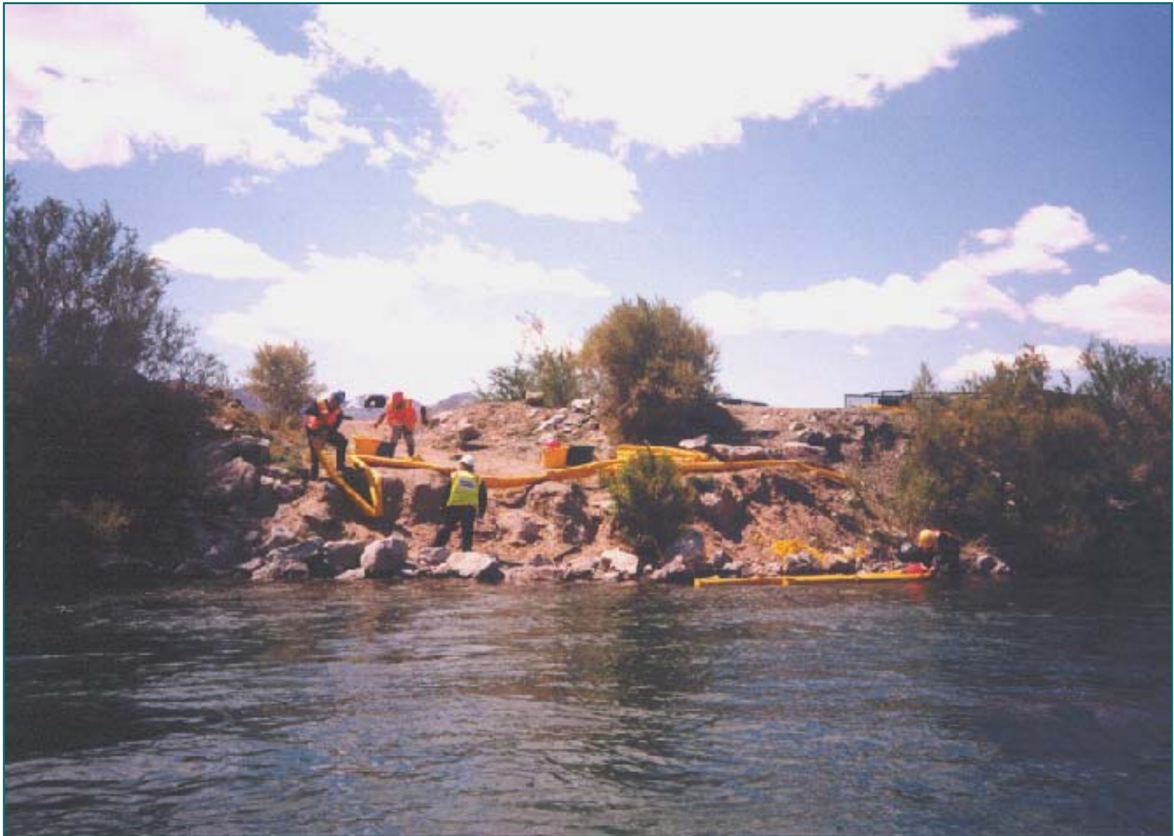
Bridge to Bank Rope Anchor System - Boom Layout on River Bank Colorado River - Nevada
