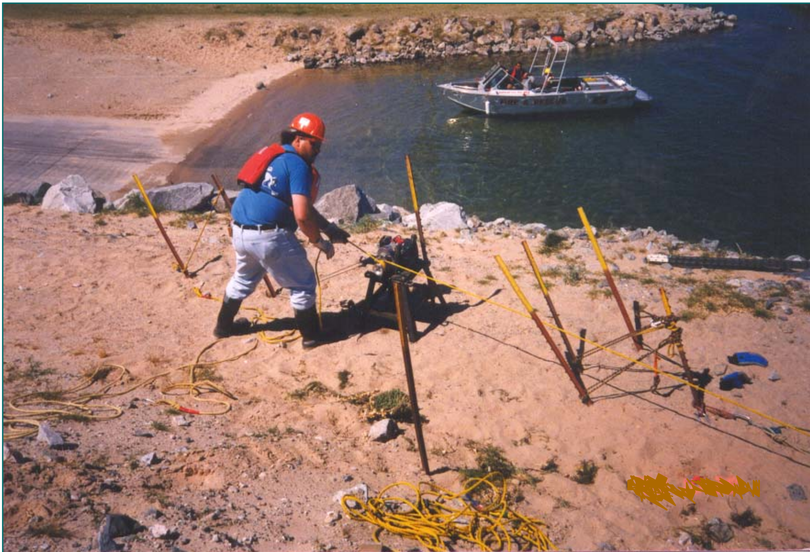
Rope Being Pulled by Power Winch with Side Capstan Mounted on Stand Colorado River - Nevada
