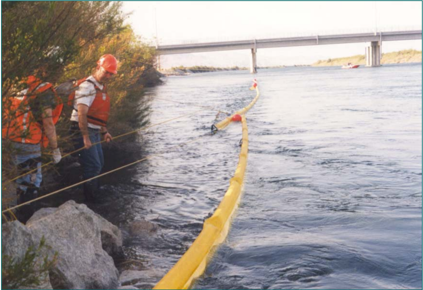
Bridge to Bank Rope Anchor System Colorado River - Nevada
