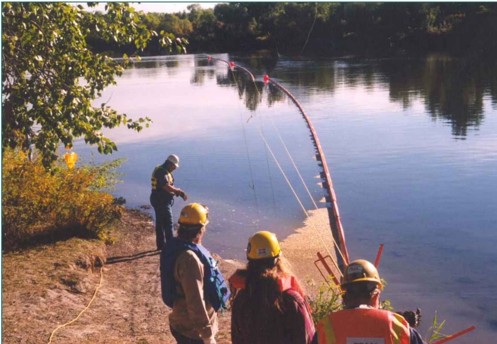
Bank to Bank Rope Anchor System Missouri River - Montana
