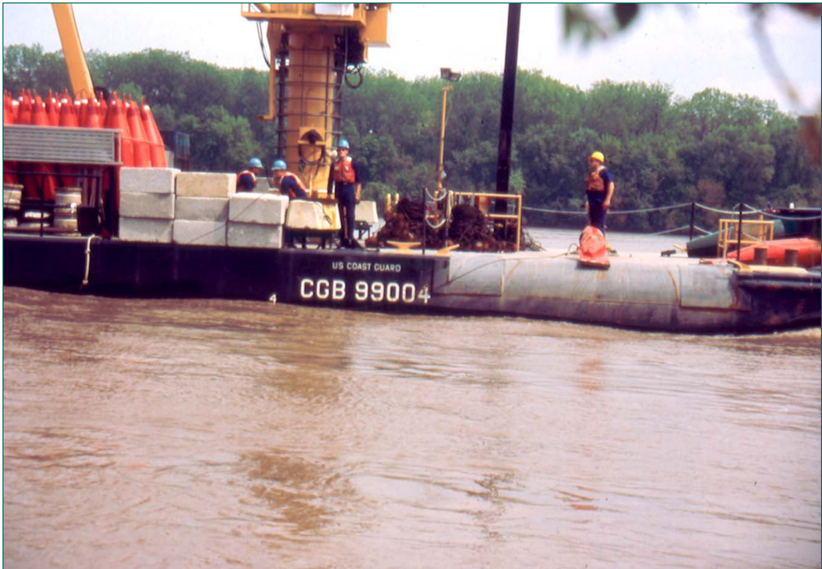
Buoy to Bank Anchor System USCG Buoy Tender in Position to Drop 1600 lbs. Sinker with Buoy Missouri River - Missouri
