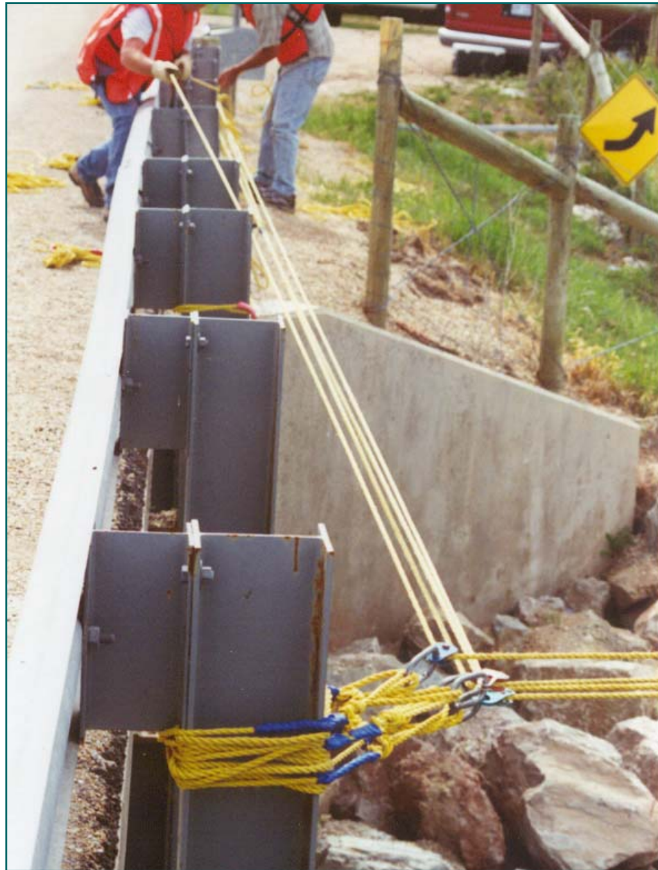
Pulley System from I-Beam
