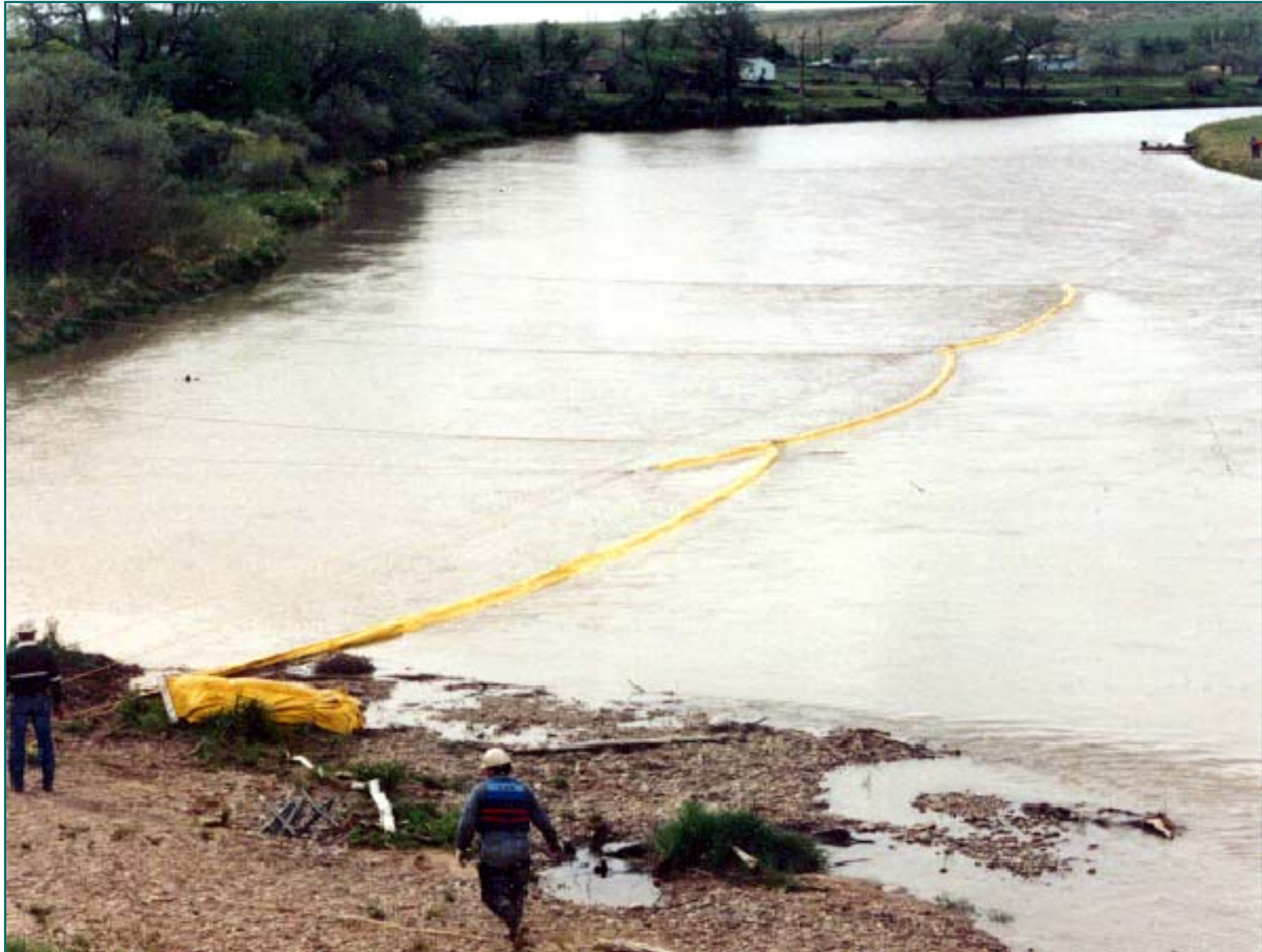
Bank to Bank Rope Anchor System Platt River - Wyoming
