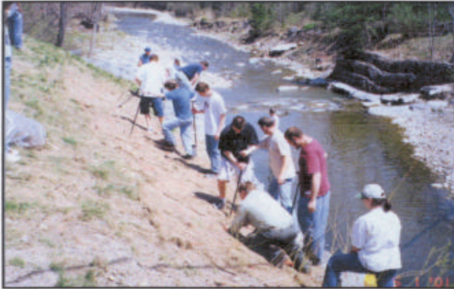
Holland High students and Erie County Department of Environment & Planning and USDA Natural Resources Conservation Service volunteers planting Red osier dogwood and Streamco willow bare-root seedlings through Geo-jute erosion control fabric, Spring 2001.
