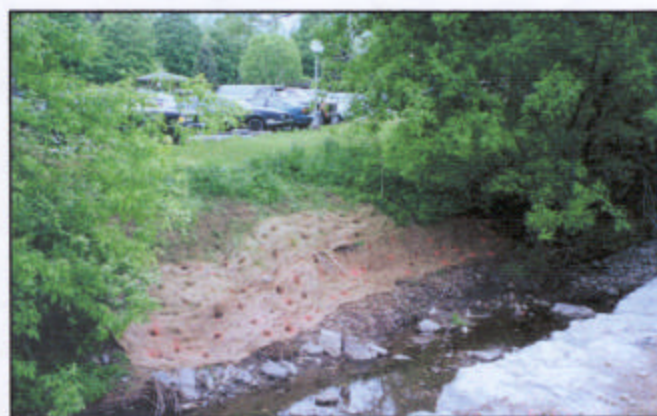
Finished bank opposite rock wall planted with Red osier dogwood and Streamco willow bare-root seedlings through Geo-jute erosion control fabric, Spring 2001.
