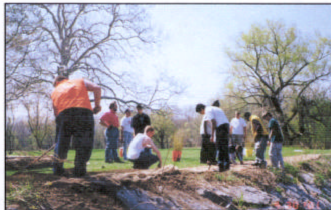
Gow School students and West Seneca AmeriCorps planting seedlings through Geo-jute erosion control fabric above the slope rock and filling in a gully (lower left), Spring 2001.
