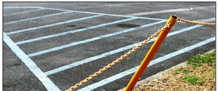
Paved areas such as parking lots and roadways can be used as caps over contaminated soil
