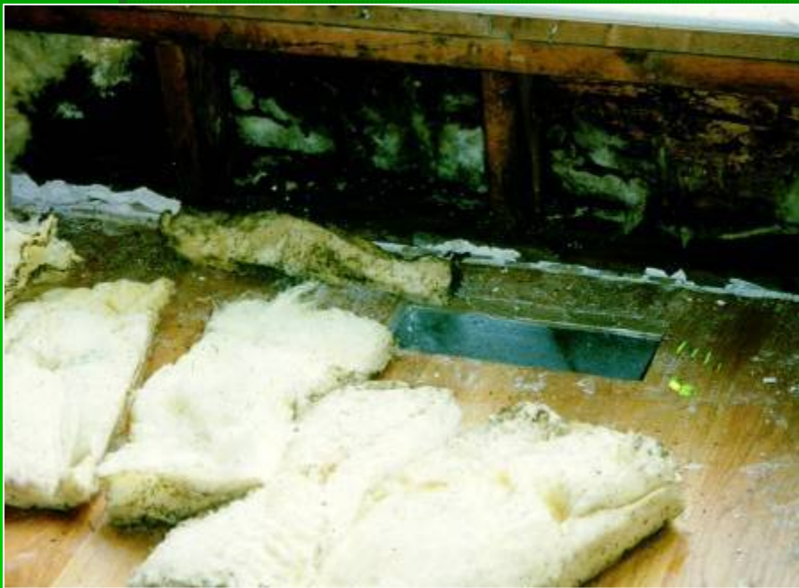
Black Mold Damage
