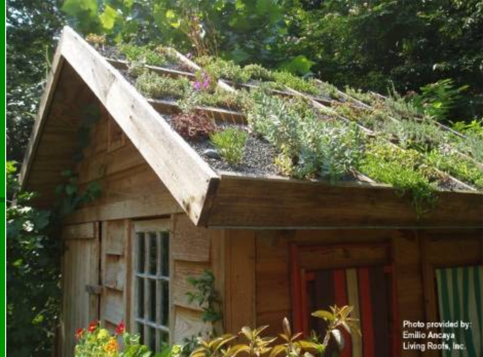
Photo from www.waterproofing.co.nz
