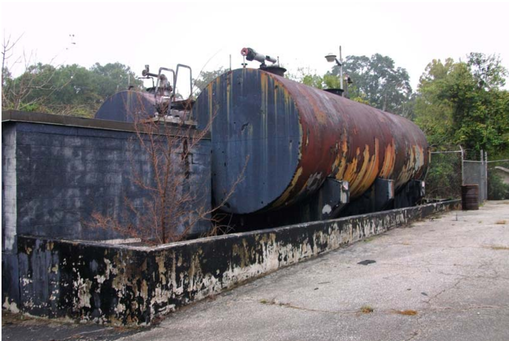
Photograph No. 7: Fuel oil storage tanks.
