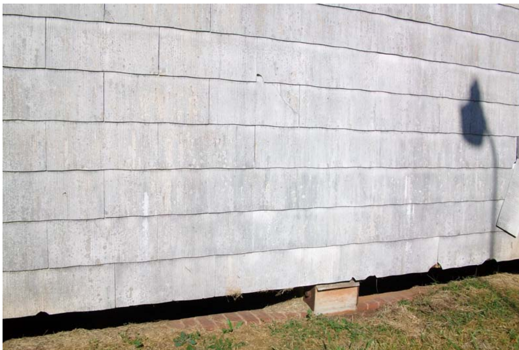
Photograph No. 2: Possible asbestos containing material (ACM) shingles on exterior of Warehouse No. 1.
