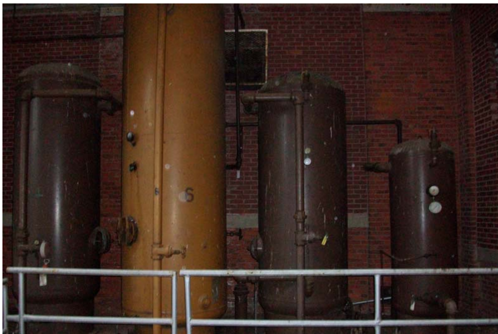
Photograph No. 6: Compressor tanks.
