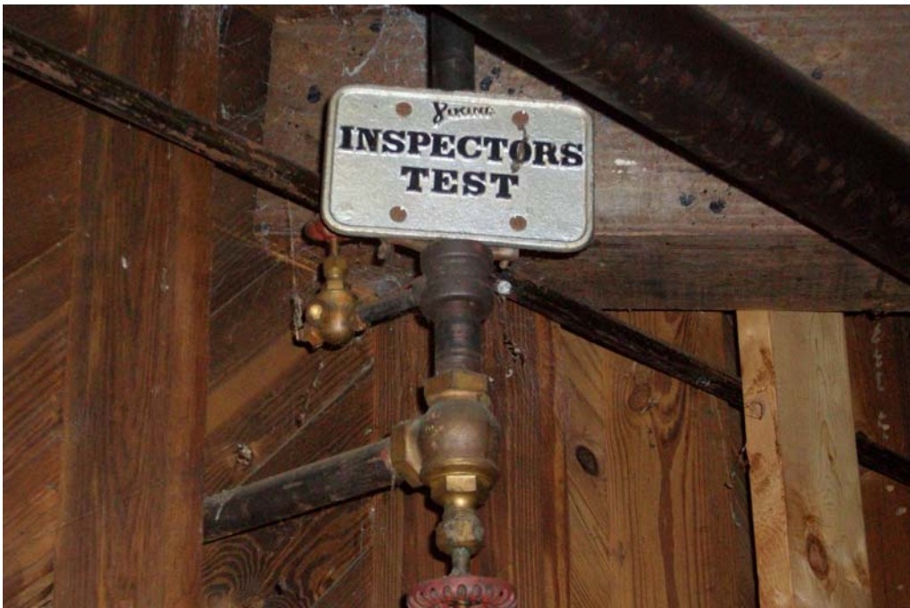
Photograph No. 8: Sprinkler system inspector test plate.
