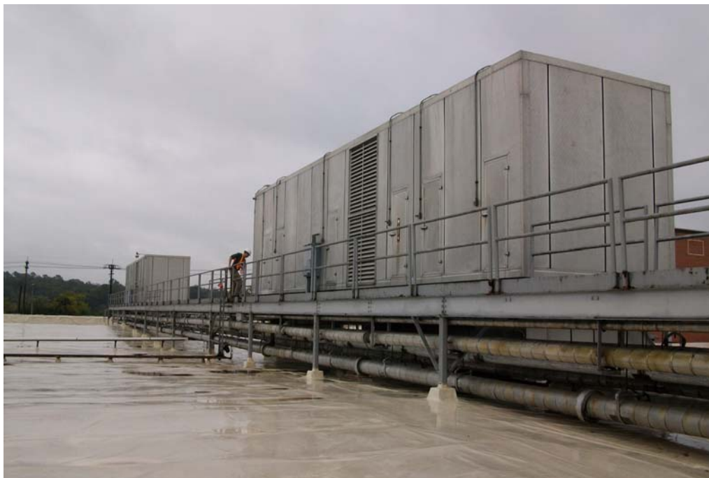
Photograph No. 1: Rooftop air handling units and associated steel support structure above Weave Room No. 2.
