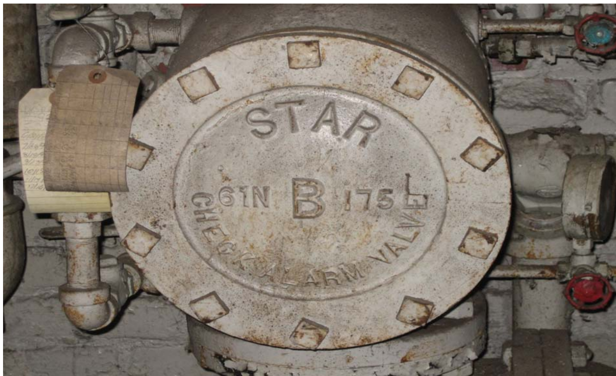
Photograph No. 6: Sprinkler system plating in Thornhill 7C
