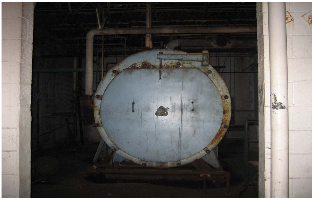
Photograph No. 4: Boiler tank in Thornhill 7D
