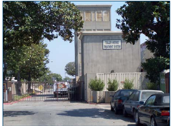
MTBE treatment at the Tuller Avenue ground water treatment system
