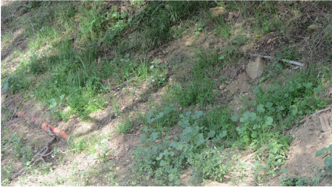
Figure 31. Exposed Water Pipes Adjacent to Fire Road, View North
