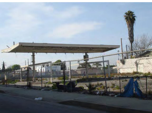
Former Kim's ARCO Station in Compton, CA, destroyed during the 1992 Los Angeles Riots.
