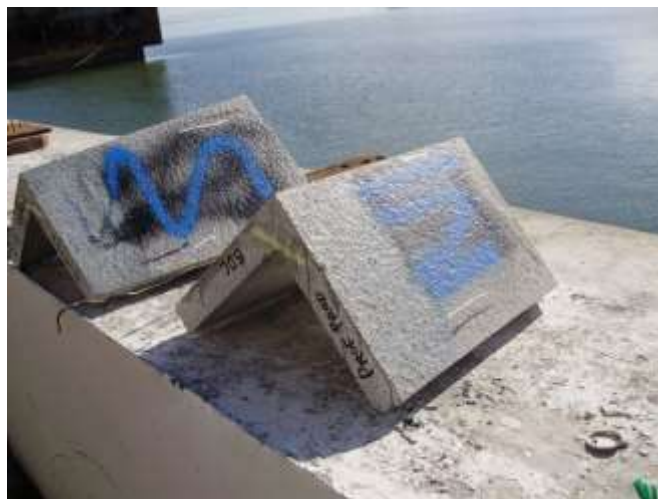
Figure 5-9. Graffiti resistant coatings on granite with graffiti
