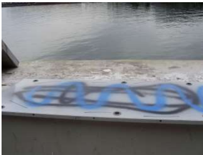
Figure 5-14. Coval coating on fiberglass panel with graffiti
