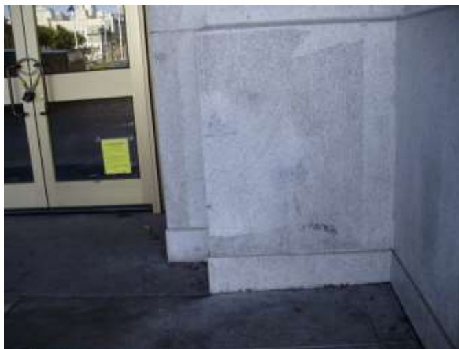
Figure 2-9. Building with graffiti resistant coating showing shadowing
