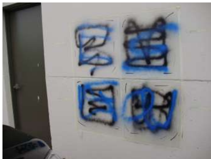
Figure 5-8. Graffiti resistant coatings on stucco wall with graffiti
